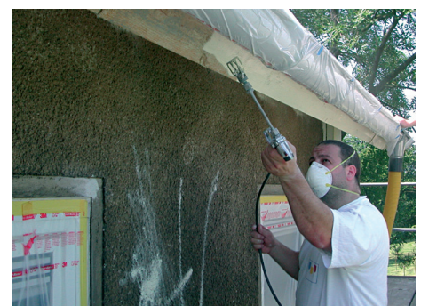
Spray painting of a cladding: neighboring parts must be protected from the resulting mist of paint.
